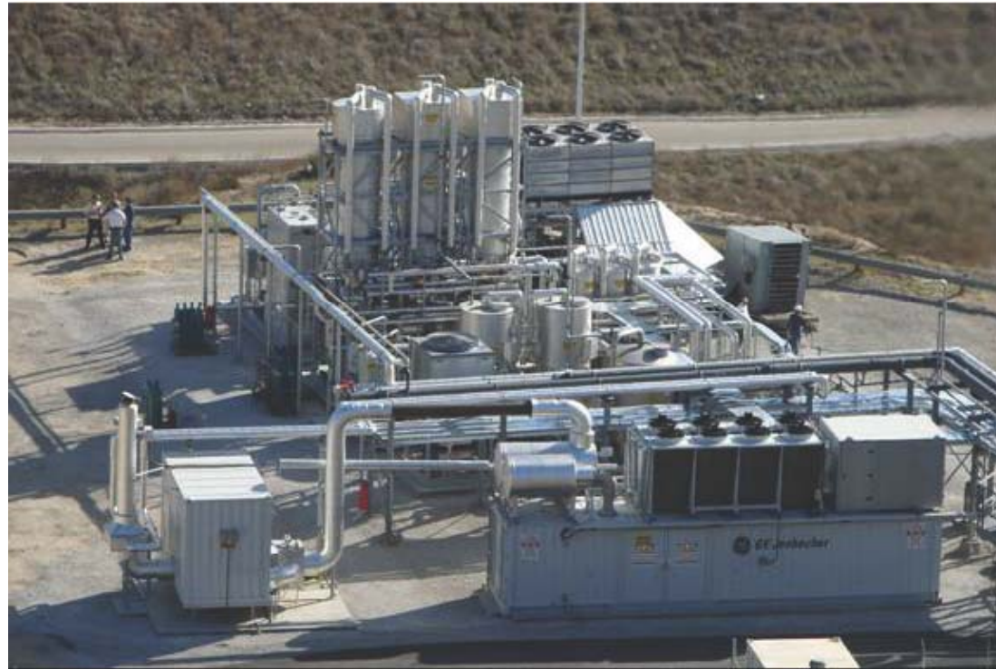
Cryogenic upgrading facilities
